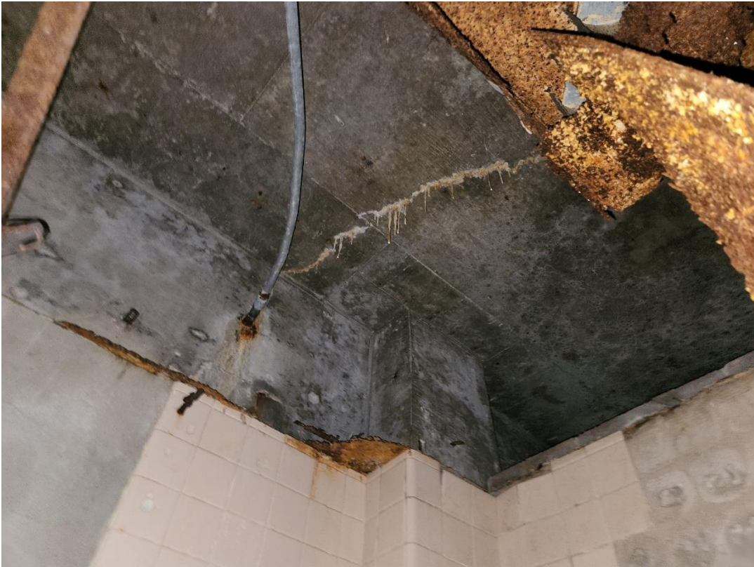
Picture 7: Crack in the concrete slab at the South Annex has allowed calcification to form.
