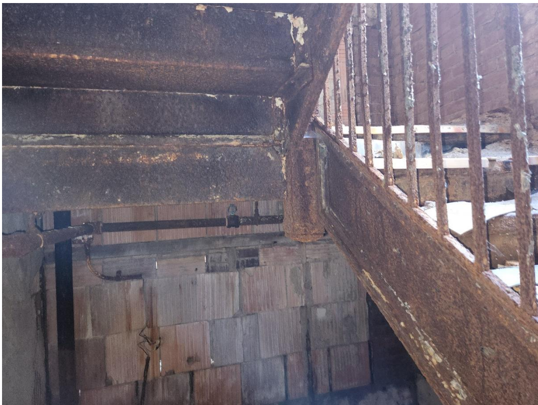
Picture 4: The steel stair structure is severely deteriorated and shall be replaced.
