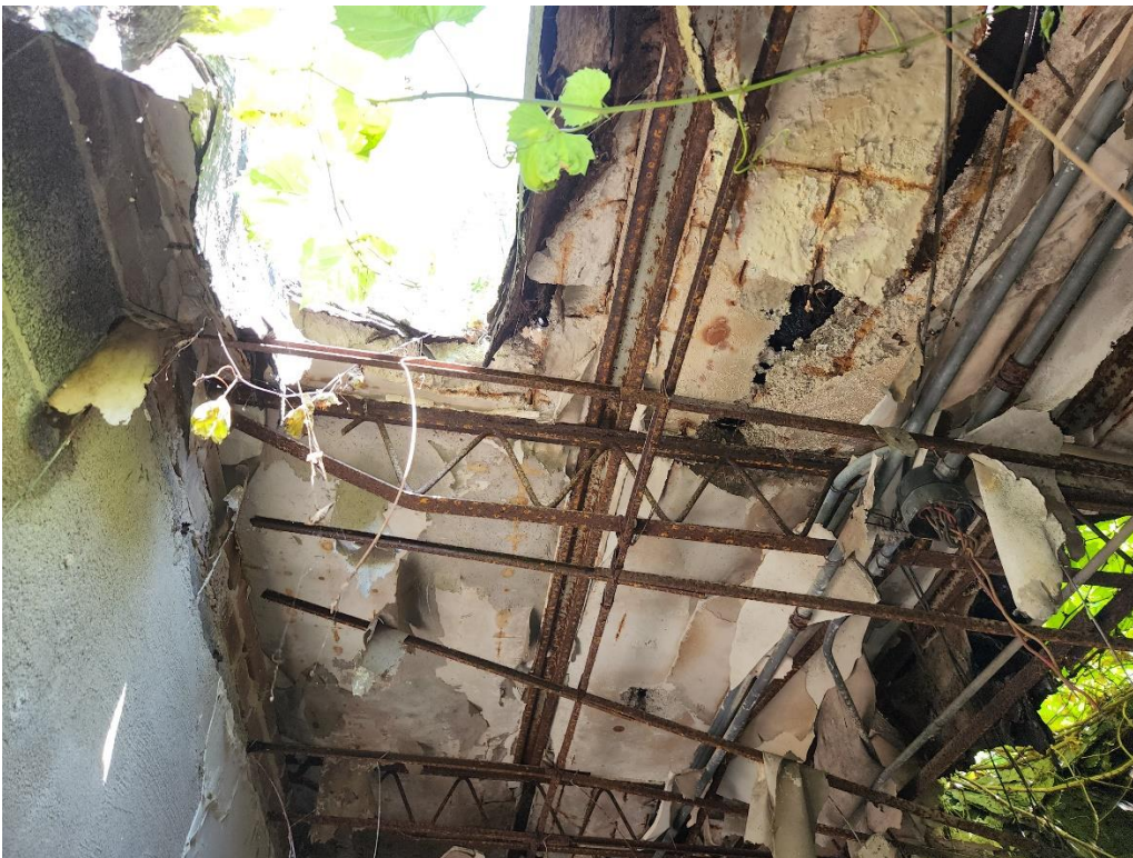
Picture 2: The West Annex roof has collapsed, exposing the structural steel to the elements, and has caused significant deterioration.
