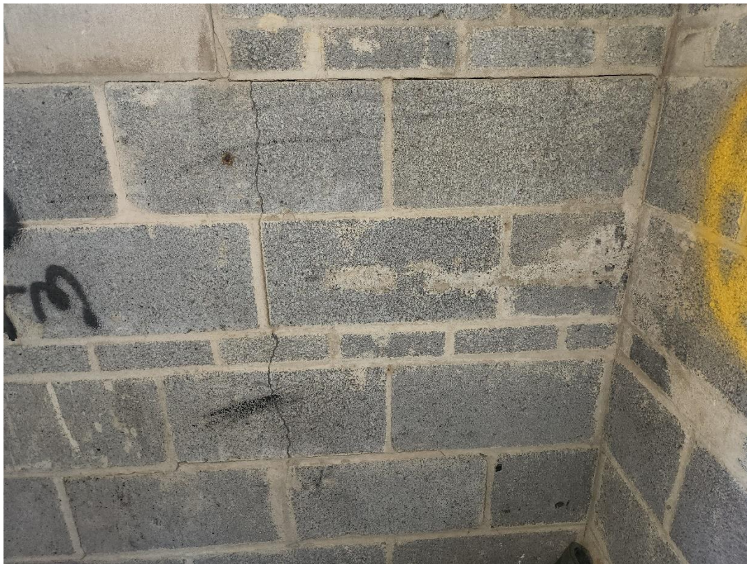
Picture 8: Cracks in the exterior concrete masonry walls at the penthouse shall be tuck pointed.
