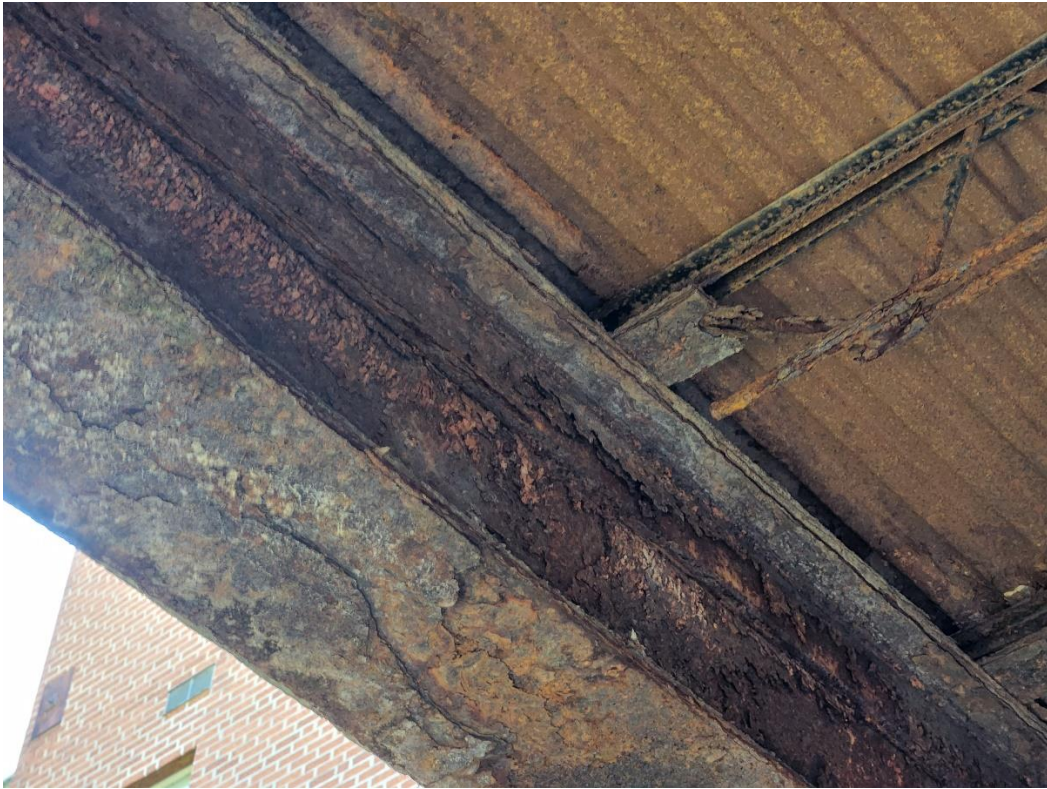
Picture 3: Steel at the exterior walkway is severely deteriorated to the point that it has delaminated.
