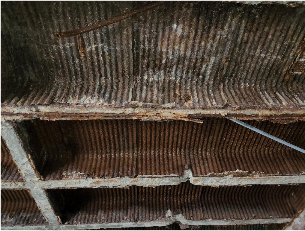
Picture 1: Concrete at the ribbed beams have cracked and exposed the reinforcement, allowing significant deterioration to occur.
