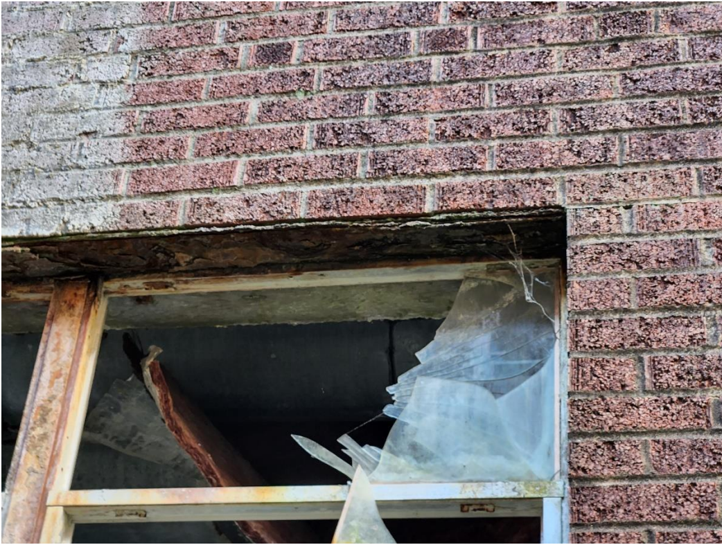
Picture 5: Exterior steel lintels are severely deteriorated and shall be replaced.
