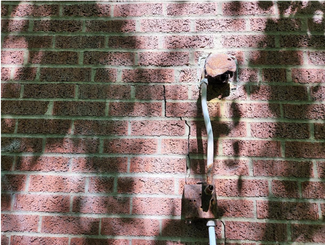
Picture 9: Cracks in the exterior brick veneer shall be tuck pointed.
